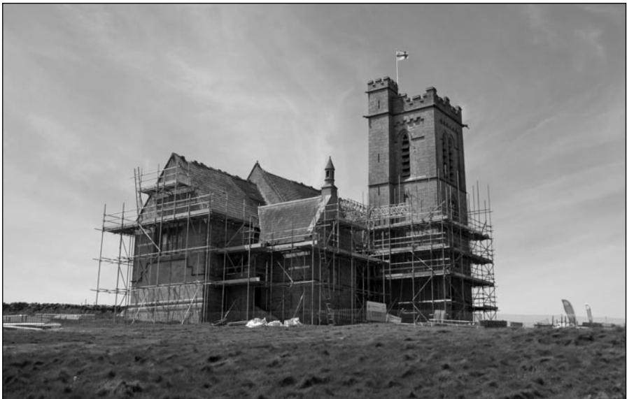
The church encased in scaffolding during the repairs and refurbishment that were undertaken in 2017. Image: Keith Hiscock.
